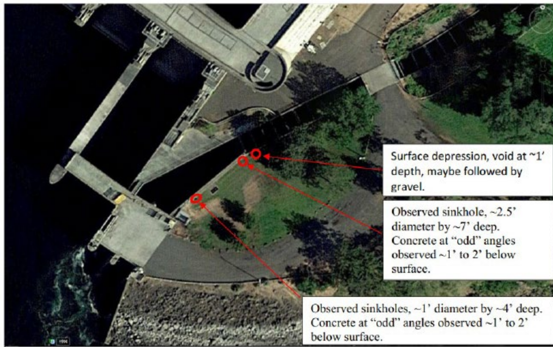
Figure 1. Aerial photo showing locations with descriptions of sink holes near The Dalles Dam west fishway entrance (south west corner of the dam).
